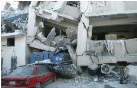
A heavily damaged building, implying that anybody in certain areas of this building were inevitably killed or trapped.
